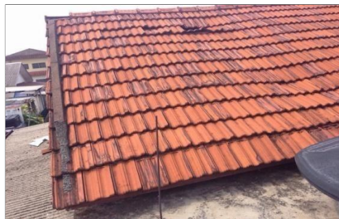
Figure 1.3 Corrugated Roof Due to Wrong Measure of Roof Trusses.
